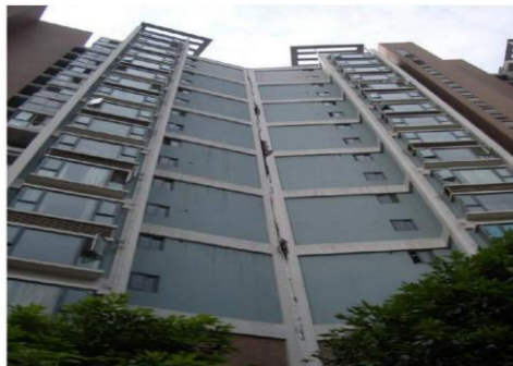
Figure 5: Pounding damage: (a) 1999 Taiwan earthquake and (b) 2008 Wenchuan earthquake (reprinted from Hao, 2015).
