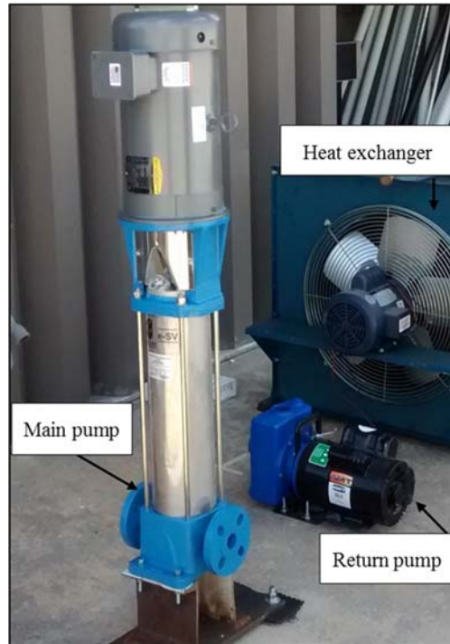
Figure 8. Photograph depicting major components of the water supply system.
