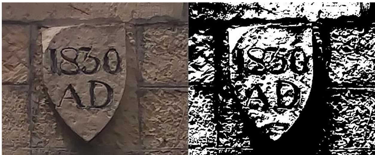
Figure 23 Keystone above a side entrance of St. Philips Church painted “1830.” Using the threshold tool in Adobe Photoshop I discovered that at some point the date was changed. The original date was “1850.”
