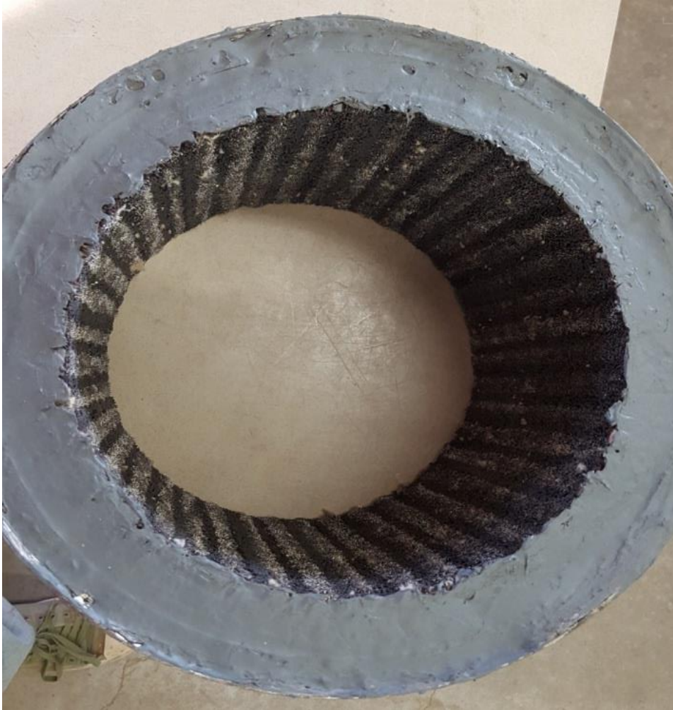
Figure 7. A finished drum coated with 3M™ Fire-Barrier Sealant Caulk CP 25WB injected into the voids in the drum and 3M Fire-Block Sealant FB136 laid over the 3M™ Fire-Barrier Sealant Caulk CP 25WB.
