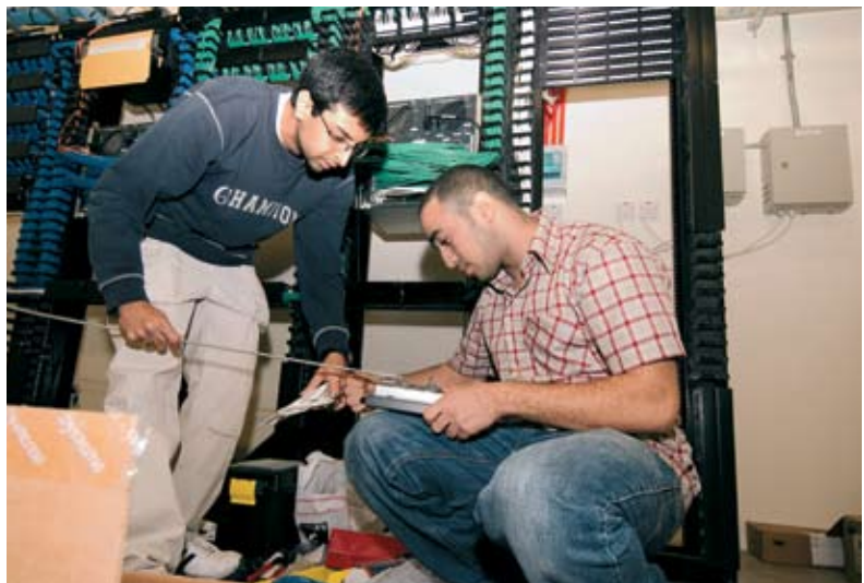
ITS student workers are continuing to help ready the building for the fall semester, seen here putting together wireless access points.
