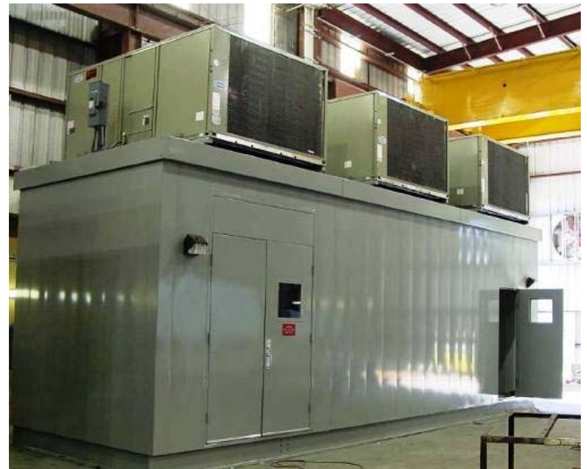
ICB / PCR for 5000 HP VFD Redundant ACU
