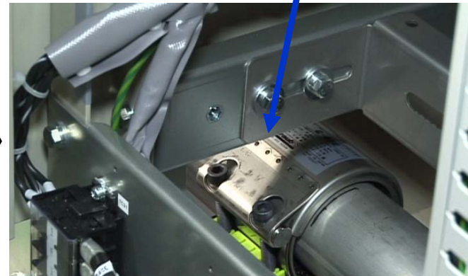
Straub Coupling between the inverter panels
