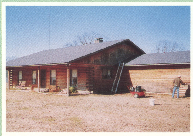
Continual maintenance is essential in order to prevent problems caused by weathering, mildew and wood decay.
