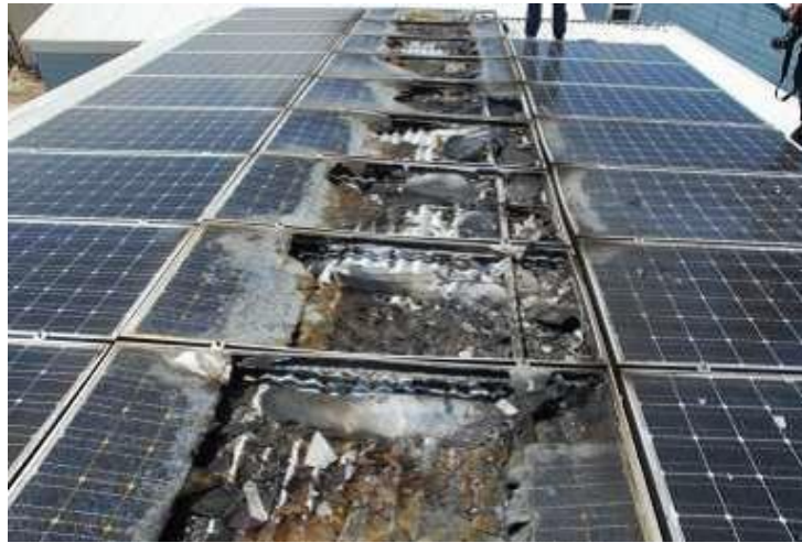
Figure 1 PV panel fire case taken from [10]
