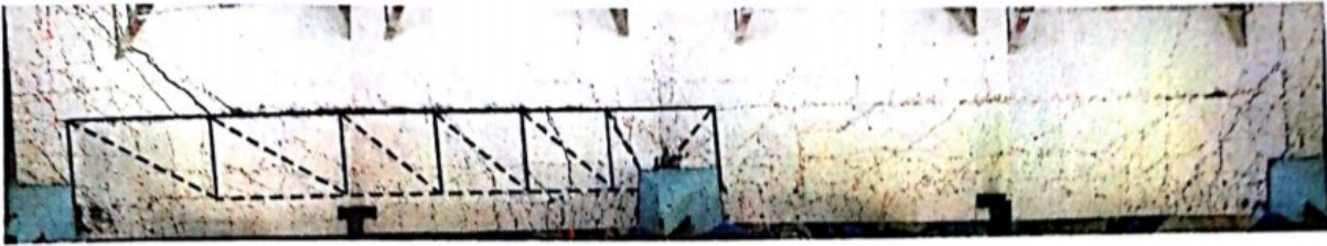
(a) Folded plate mechanism evident due to crack patterns in the infill region.
