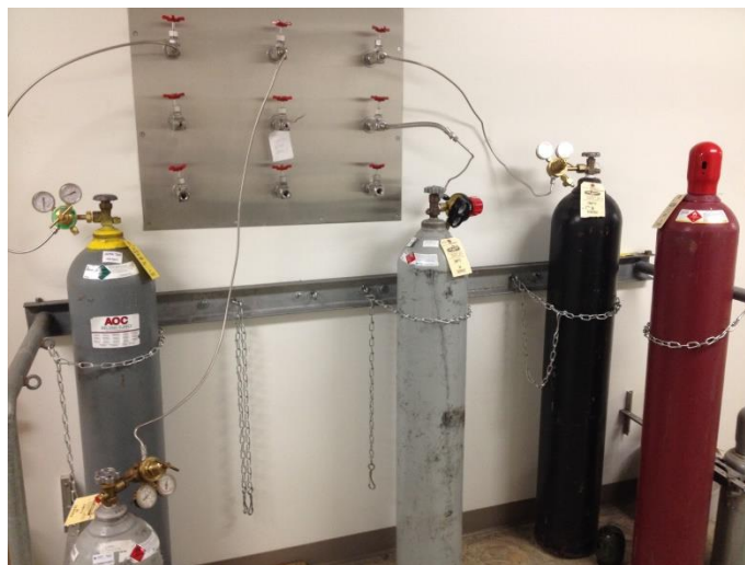
Figure 11 Chemical supply (Pressurized cylinders) and the wall panel valve
