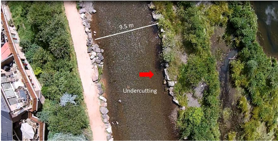
Figure 24: UAV video (screenshot) (2014) depicting undercutting banks.
