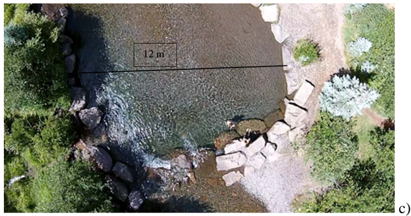
Figure 26: Drop Structure directly downstream of Pacific Avenue Bridge: a) 2002 a year after construction; b) Eastern side starting to fail in 2004; c) Grade control has minimal effect, Screenshot of UAV video, 2014.
