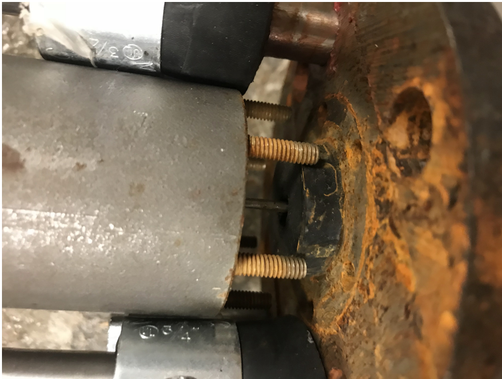
Figure 3.11: Oxidation on the inside of the Pipe and end cap
