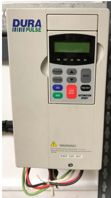
Figure 2.17: Automation Direct VFD used for experiments.
