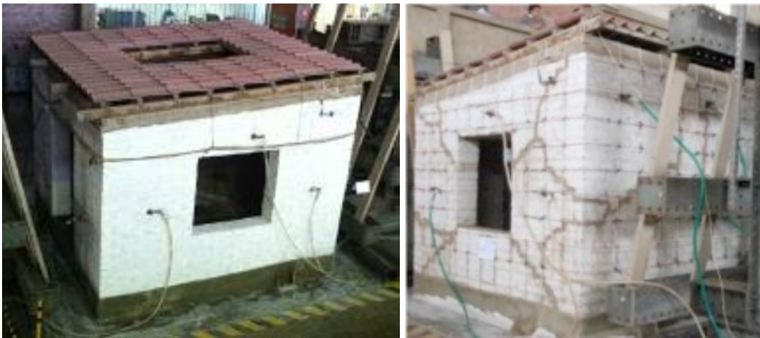
Figure 3.1. One-story adobe building. Left. Building before first seismic test. Right. Damaged building (retrofitted) ready for second seismic test (Reprinted from Blondet et al. 2017).
