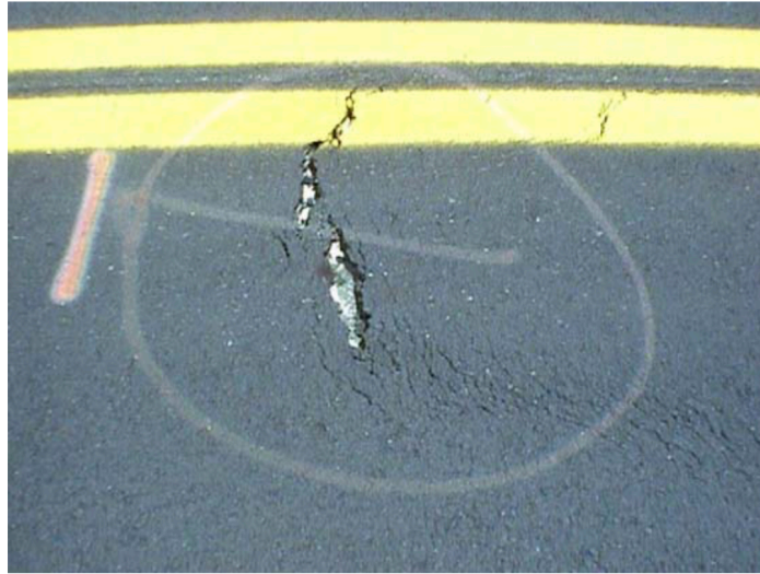
Figure 6. Cracking and Delamination on CR 315 (Reprinted from Sholar et al., 2002)
