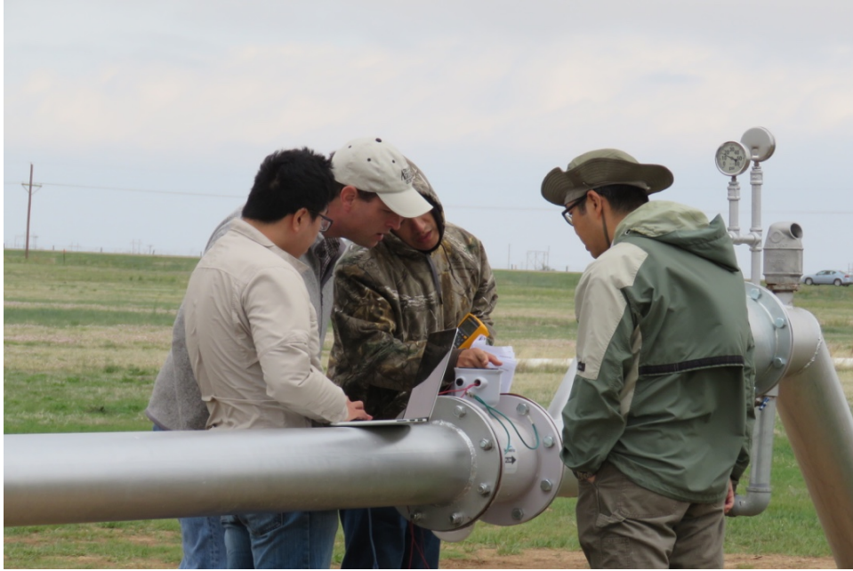
Figure 5.4: A digital flow meter is installed and connected to the control center.
