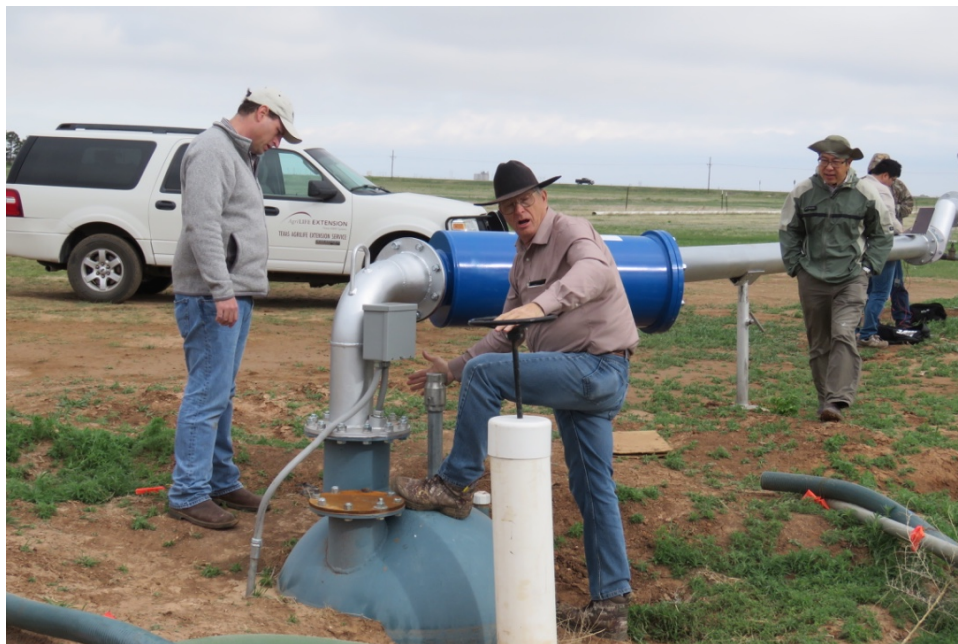
Figure 5.3: Water is pumped from a local reservoir through underground pipeline to the pivot. Mr. Marek was controlling the water flow through a valve.
