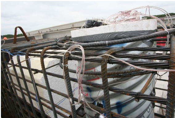
(b) PSV-28B Strain Gauged Mild Steel Shear reinforcement, Mild Steel Hoops, and Corrugated Steel Pipe
