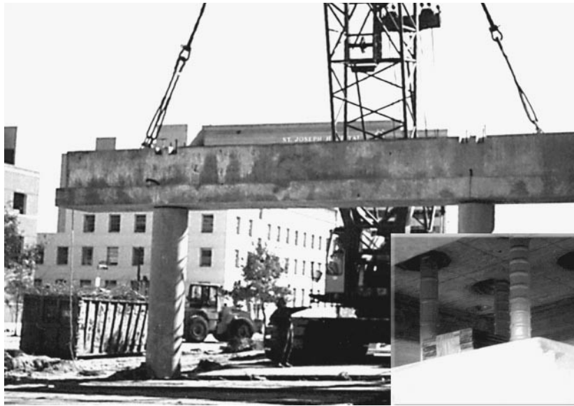
Figure 2.1. Pierce Elevated Precast Concrete Bent Cap and Beam-Column Connection (Jones and Vogel 2001).
