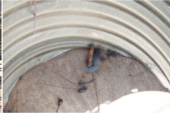
(b) PSV-28B Welded Metal Tabs Securing Corrugated Pipe
