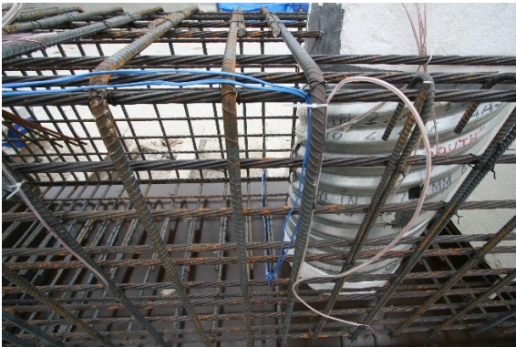
(a) PSV-28A Strain Gauged Mild Steel Shear Reinforcement and Corrugated Steel Pipe
