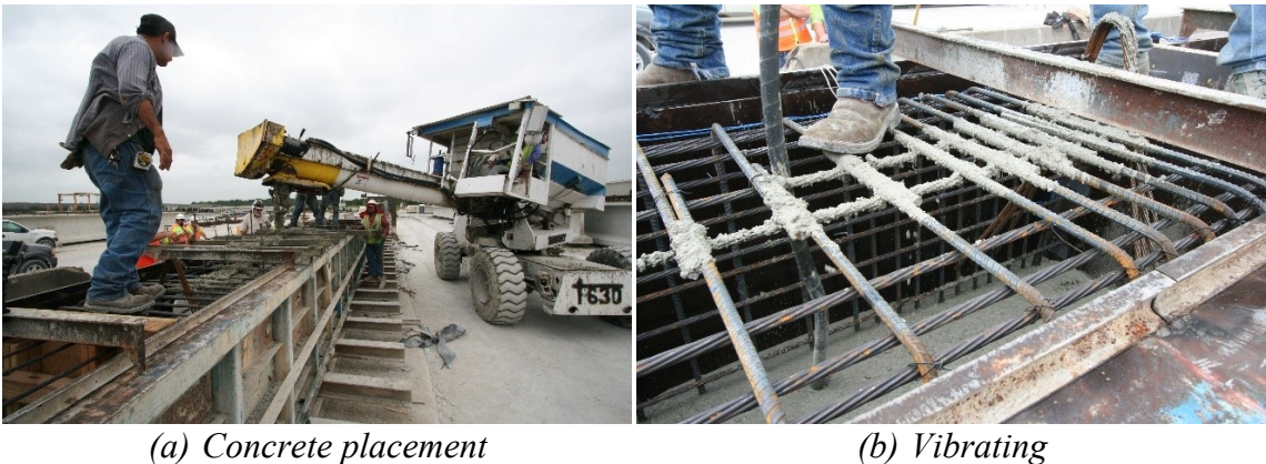
Figure 3.30. Concrete Placement and Consolidation. (Reprinted with permission from Birely et al. 2018a)
