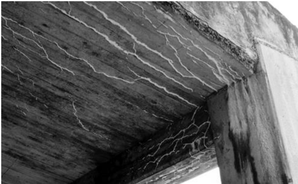
Figure 5 – White calcium carbonate traces at concrete surface, indicating autogenous healing of cracks reprinted from [22].
