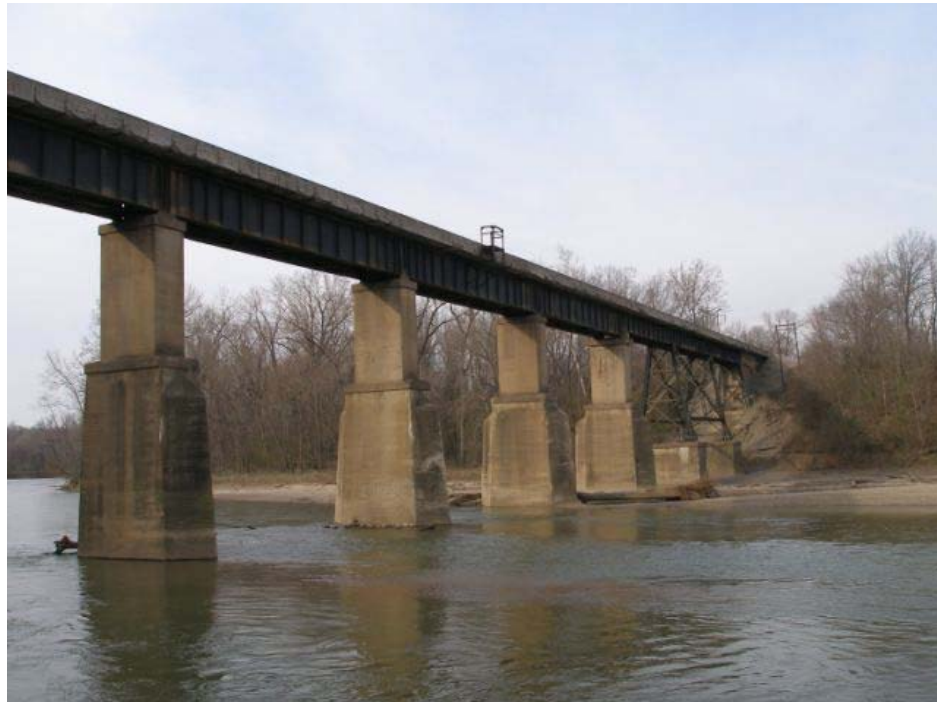
Figure 7-3 Vintage riveted steel girder span in revenue service. Reprinted with permission from Otter et al. [14].
