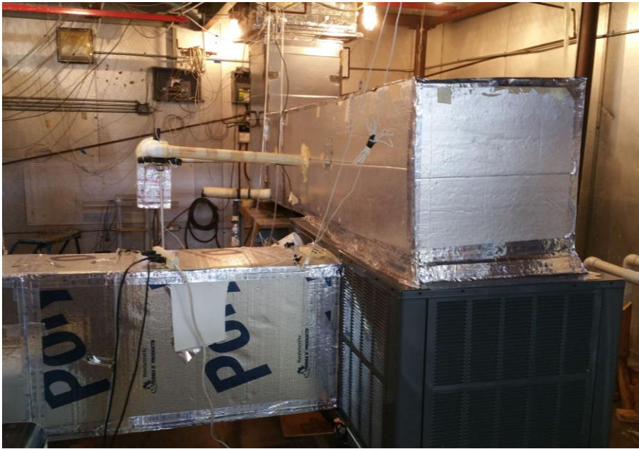
Figure 8: HVAC unit installed in the psychometric station before the integration of an evaporator cooler.
