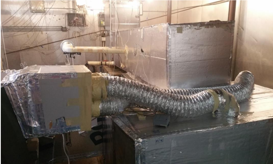
Figure 9: Evaporative cooler being integrated onto an HVAC system.
