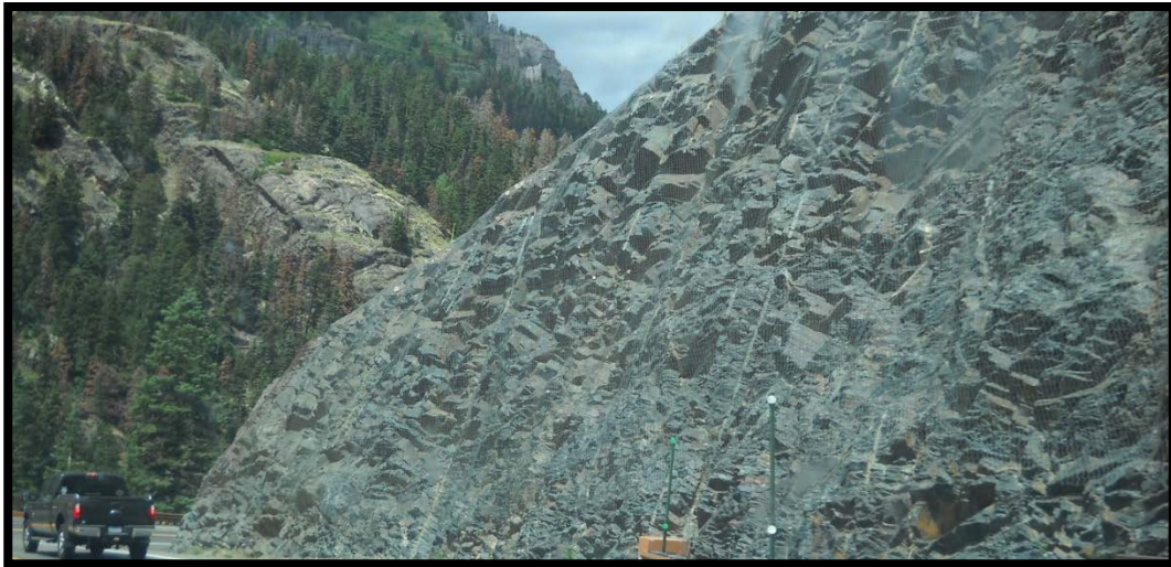
Figure C-2: Image of rock mesh installed on U.S. Highway 550 to prevent rockfall (08/07/15).
