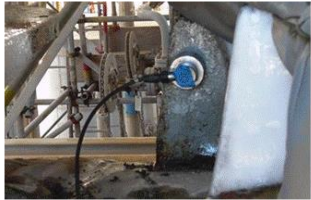
Figure 37. Velocity probe installed near piping flange on the PR compressor of Train #1
