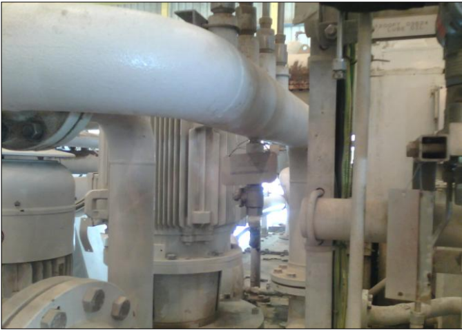
Figure 27 Secondary Sampling Port for Steam Turbine Lube Oil
