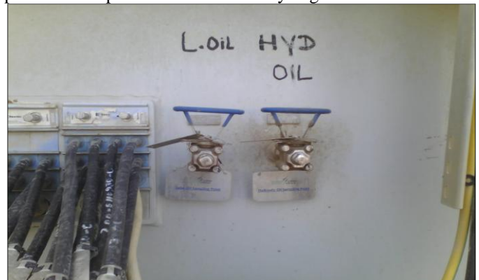
Figure 26 Primary Sampling Port for a GT Lube Oil & Hydraulic Oil
