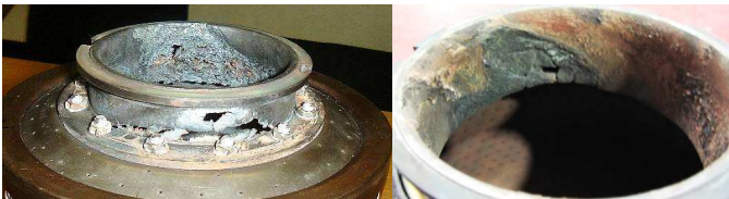
Figure 12: DLE Pre-chamber damage as the result of heavy hydrocarbon carry over and oxidation
