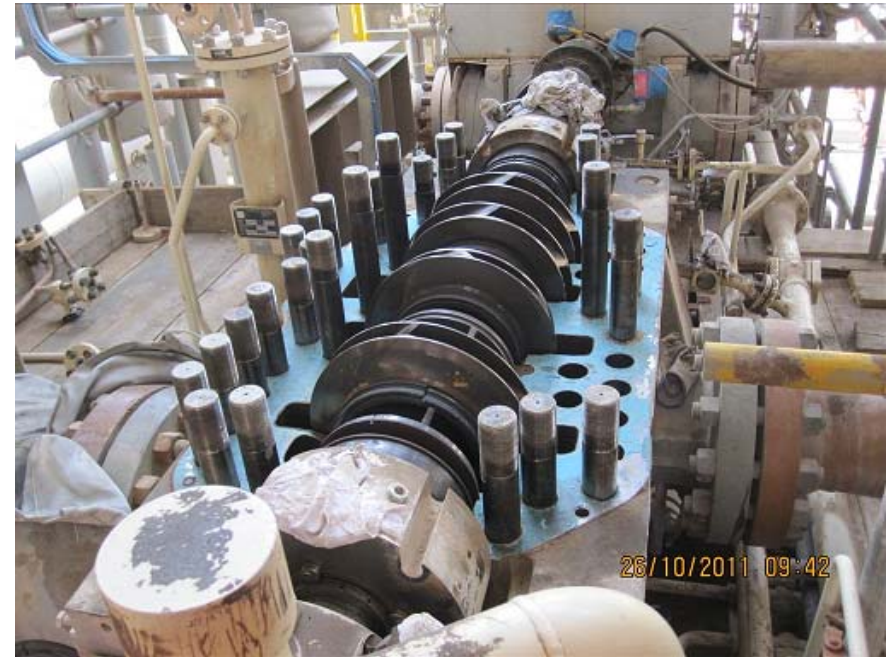
Old pump at skid in RGX2
