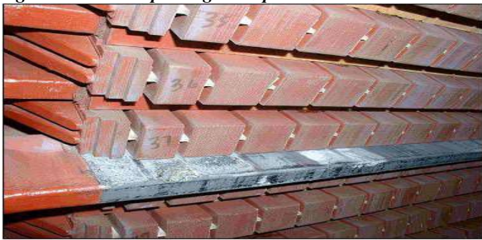
Fig. 3 – Complete winding insulation became destroyed at another power plant suspected to have similar problem.
