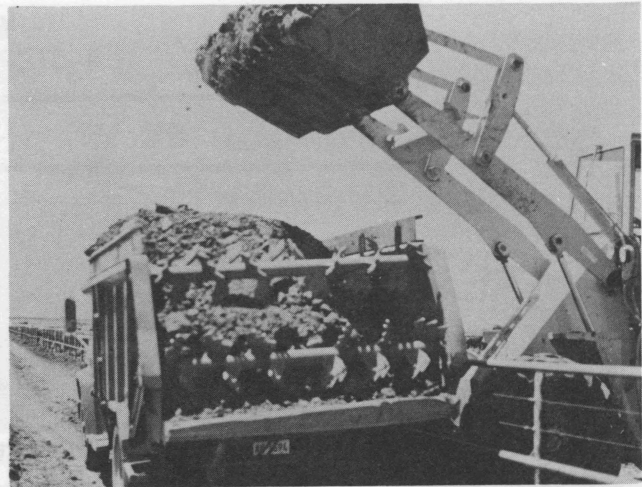
Figure 5. Nonproductive time awaiting truck arrival often detracts from the 200 tons per hour loading rate achievable with wheel loaders.
