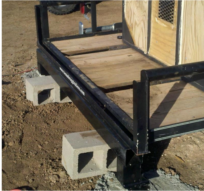
Figure 14. Constructed frame and piers used to secure on side of the trailer holding the spectrometer.
