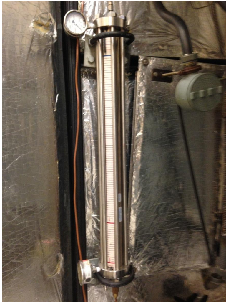
Figure 29. FPS system used in the MSD
