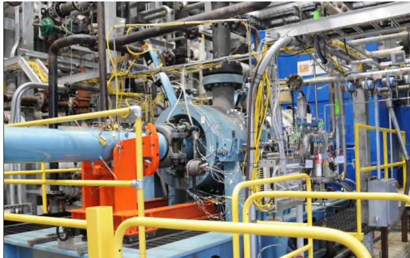
Figure 11. CO 2 compressor on test stand.
