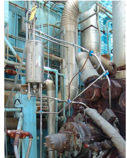
Figure 1 Piping Plan 23 in the field
