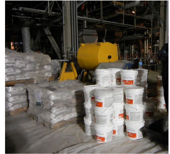
Insufficient work space for materials, mixer and additional personnel
