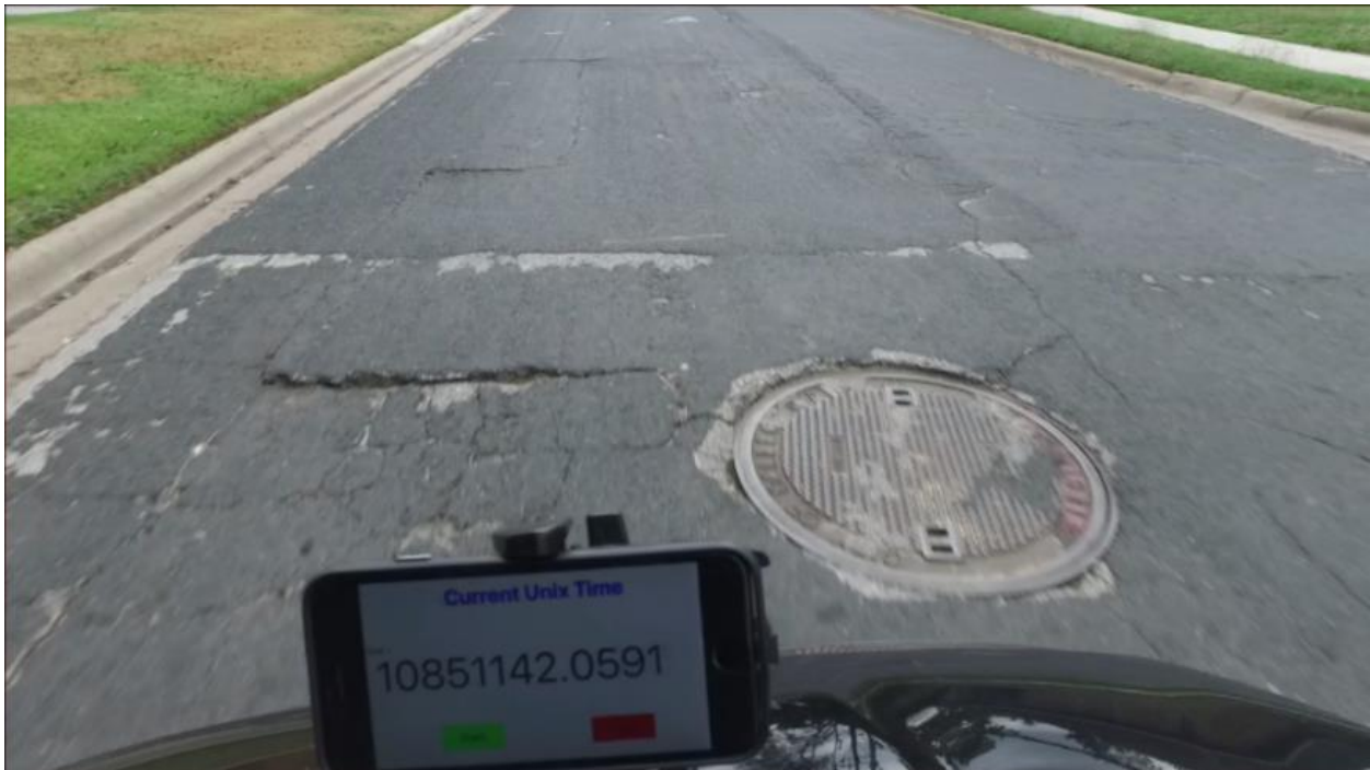
Figure 3. A frame shot with the Osmo showing a crack
