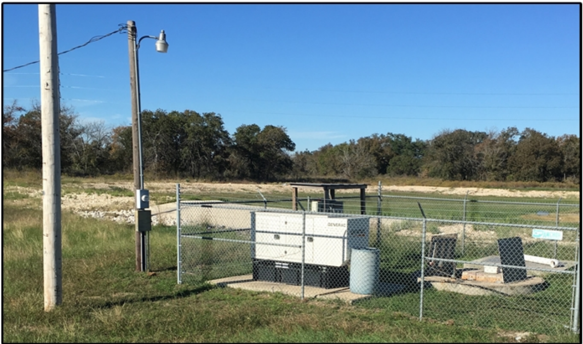
Figure 6. Lift Station at Beginning of Survey
