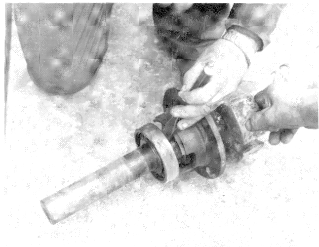
Figure 15. Questionable Procedure for Removing Rolling Element Bearings (Pump Inboard Side).
