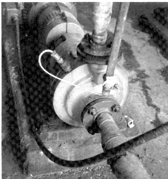
Figure 5. Pump with Sensor Mounted for Continuous Monitoring.
