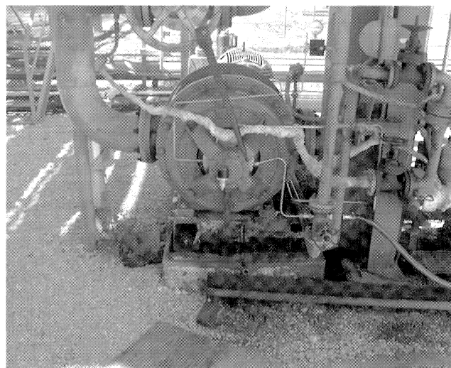
Figure 13. Nash Compressors (After PAS Was Installed).
