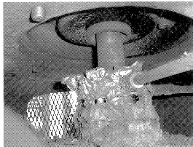
Figure 11. PAS Coated in Soot, but Leak Free after 18 Months in Service.
