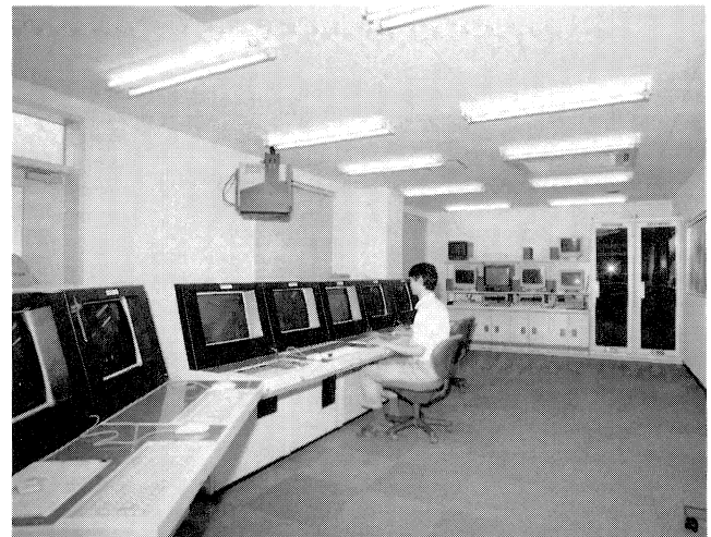
Figure 10. Pump Model Test Facility Utilizing Multimedia System.
