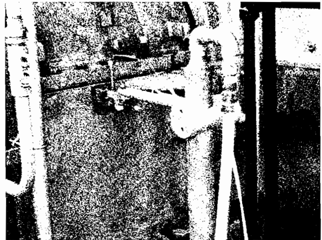
Figure 5. Water Stand and Probes Setup Early to Check the Pipe Stress Movement in the Flanging-Up Stage and the Heating-Up Stage to the TT Valve on a Front Bearing of a 30,000 HP Turbine.
