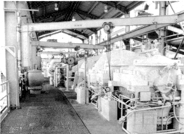
Figure 11. Compressor Floor Lifting Davits.
