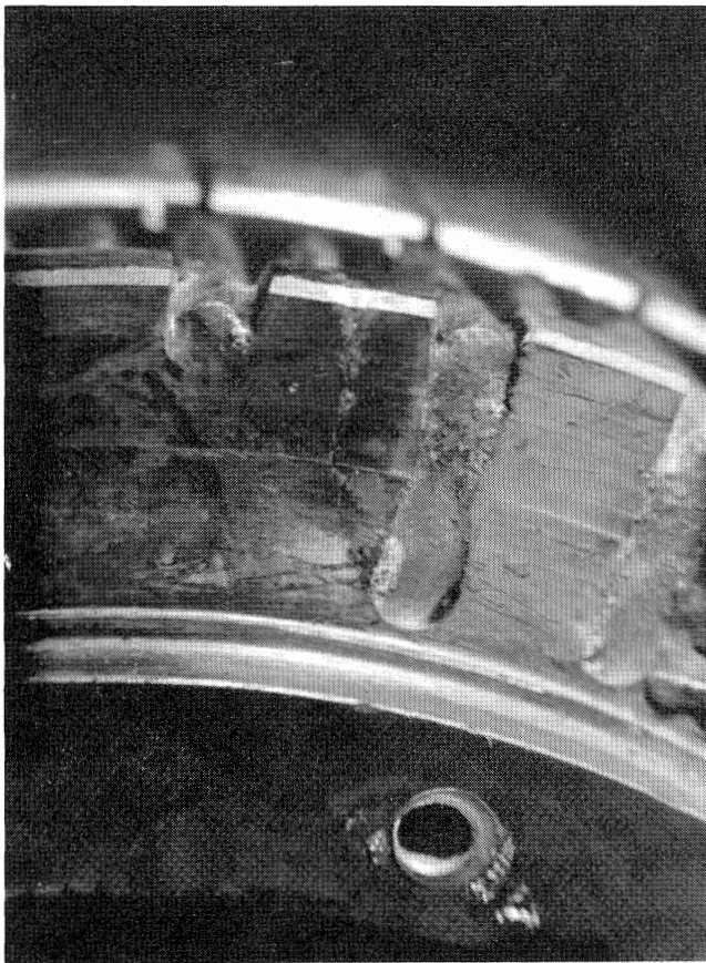
Figure 6. View of Crack in Rotor End Ring after Motor was Disassembled at Service Shop.
