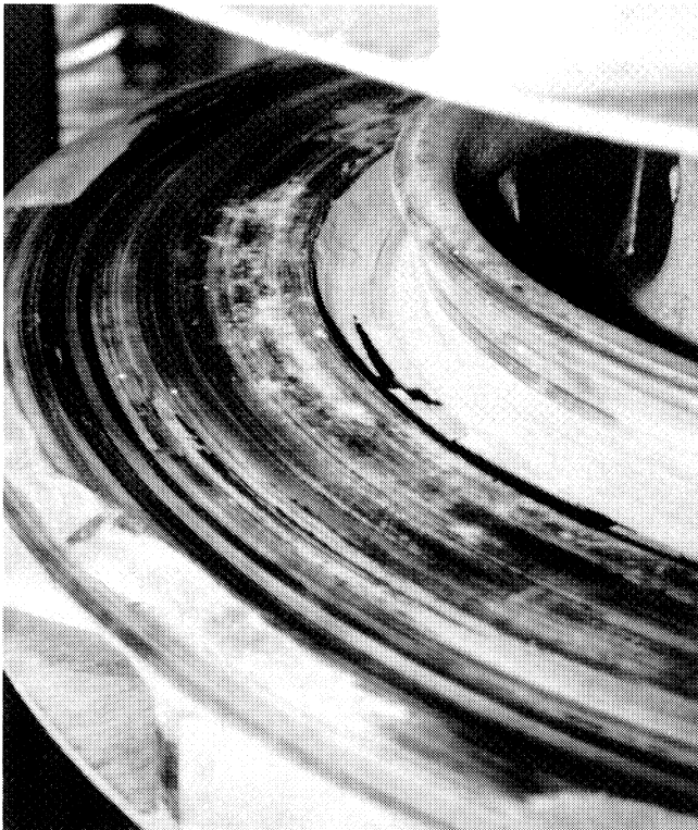
Figure 5. This Multistage Wheel Rubbed on the Upstream Diaphragm. A three in section up to one in deep was machined off the cover at the eye. The repair will include insert of a new forged cover section at the eye.
