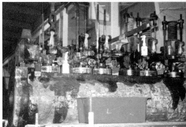
Figure 20. View of Valve Rack. Final.
