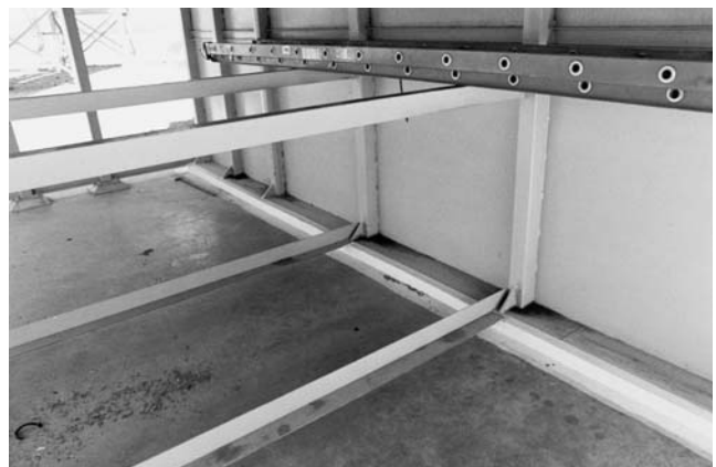
Figure 29. Filter House Where Foundation Bolts Are Missing.
