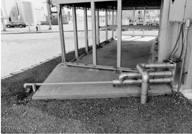
Figure 25. Drain and Overflow Piping without a Seal Leg.
