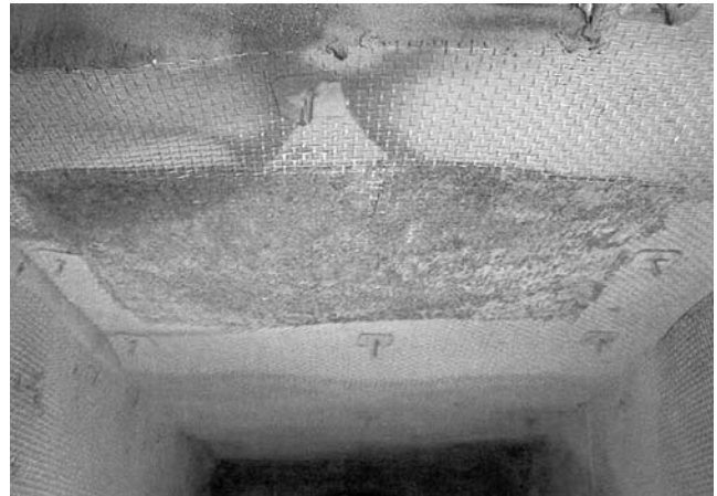
Figure 32. Location Where the Vertical Duct Enters the Horizontal Duct—Wire Mesh is a Perfect Place for Buildup of Dust. (Courtesy J. Gunsett, Yuba City Cogeneration)
