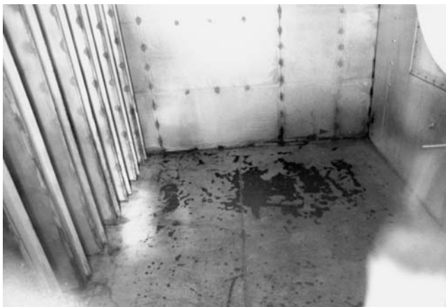
Figure 26. Floor of a Filter House with Paint Damage Caused by a Lack of Drainage.
