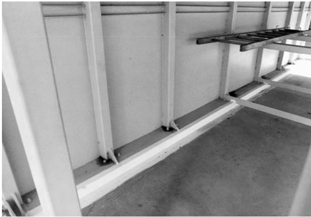
Figure 30. Sister Unit with Foundation Bolts.
