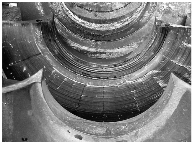
Figure 26. Damaged Inlet Guide Vanes/Diaphragms.
