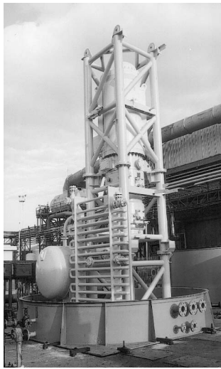
Figure 1. 850 KW (1139.87 HP) Subsea Compressor Module Refurbishment.
