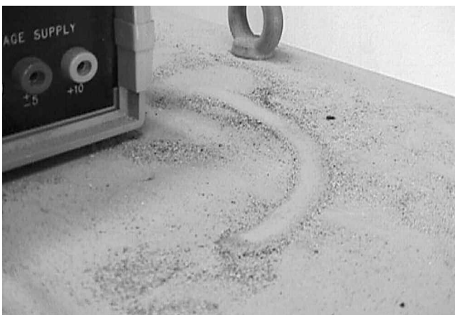
Figure 6. Sand and Dirt on Top of Magnetic Bearing Control Cabinet.
