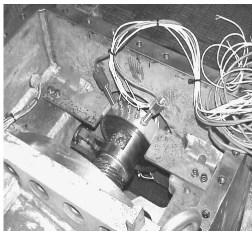
Figure 4. Top Half of Bracket with Sensors Installed.
