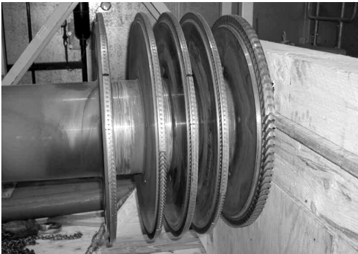
Figure 16. Turbine Rotor (Incident 1).
