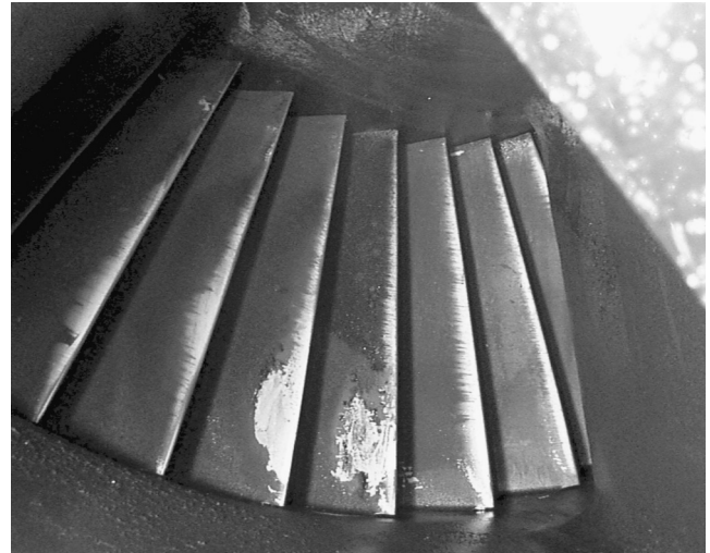
Figure 6. Fouled Compressor Blading with a Mixture of Salts and Oily Deposits.
