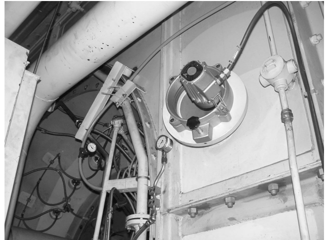
Figure 41. Illuminated Viewing Window on a 123 MW Gas Turbine.
