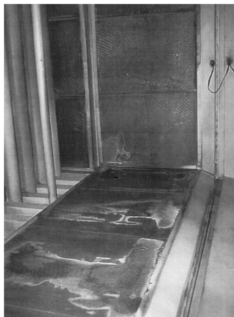
Figure 30. Corroded Floor in Inlet Duct of Large Gas Turbine.
