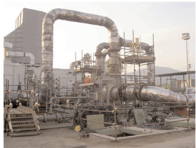
Figure 4. Test Loop Around Turboexpander Compressor.
