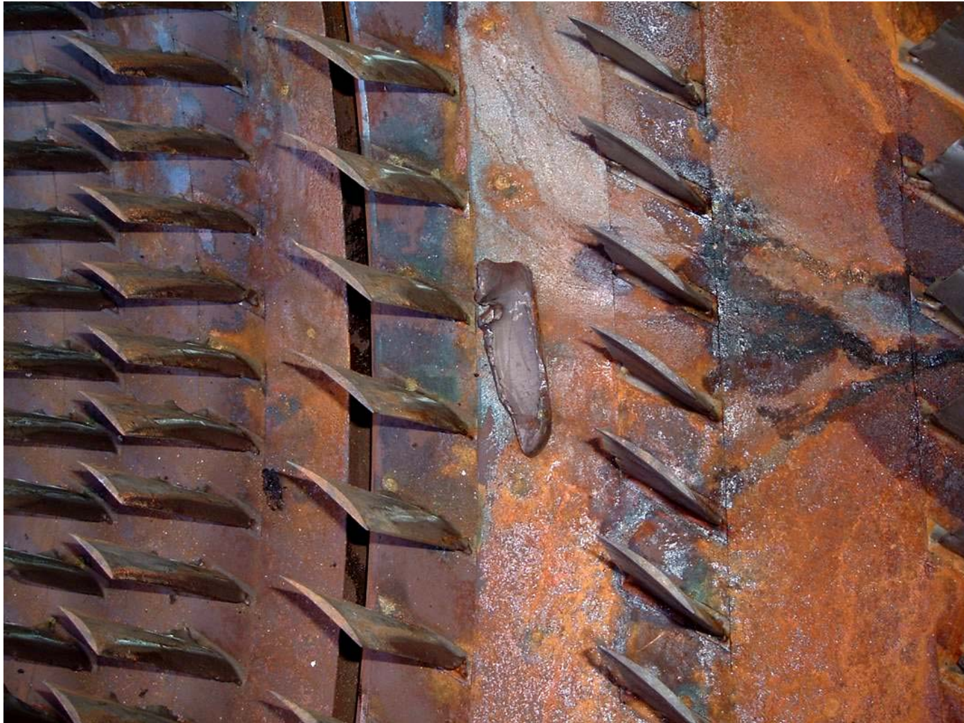
Photo of compressor stationary blading (lower half) showing a piece of a blade severed from the first stage failed blades
